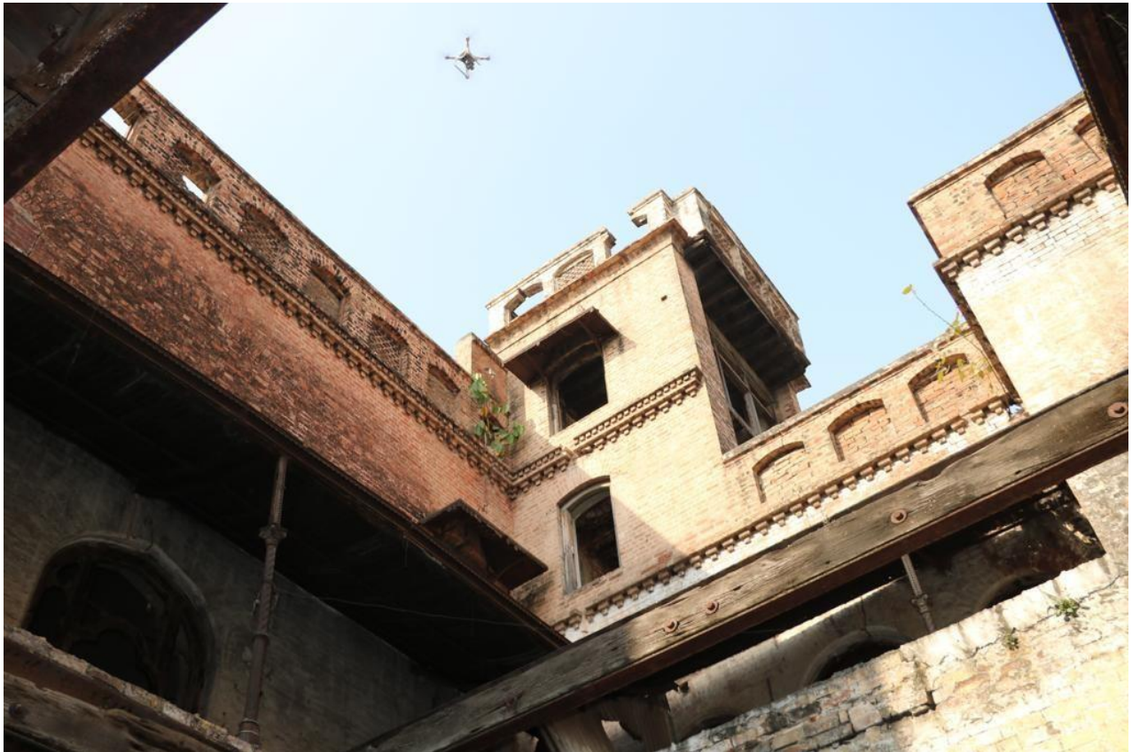
Figure 50: Worm's eye view from the Courtyard, top room 307. (Courtesy: (By F. Khan), (2018). Feroza Khan 23 Blogspot. http://ferozakhan23.blogspot.com/2018/05/ )
