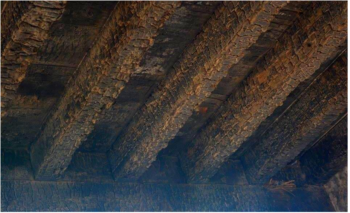
Figure 55: Wooden ceiling girders. (Courtesy: Rogers Kolachi Khan & Associates (Ltd.), Assessment of the Existing Condition at the Historic Haveli Sujan Singh, Rawalpindi, Pakistan ).
