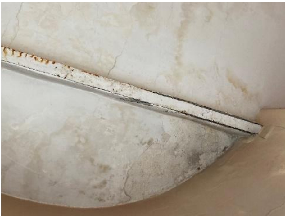
Figure 3.31. Oxidation in steel beam, Third Floor (Author, 2021)
