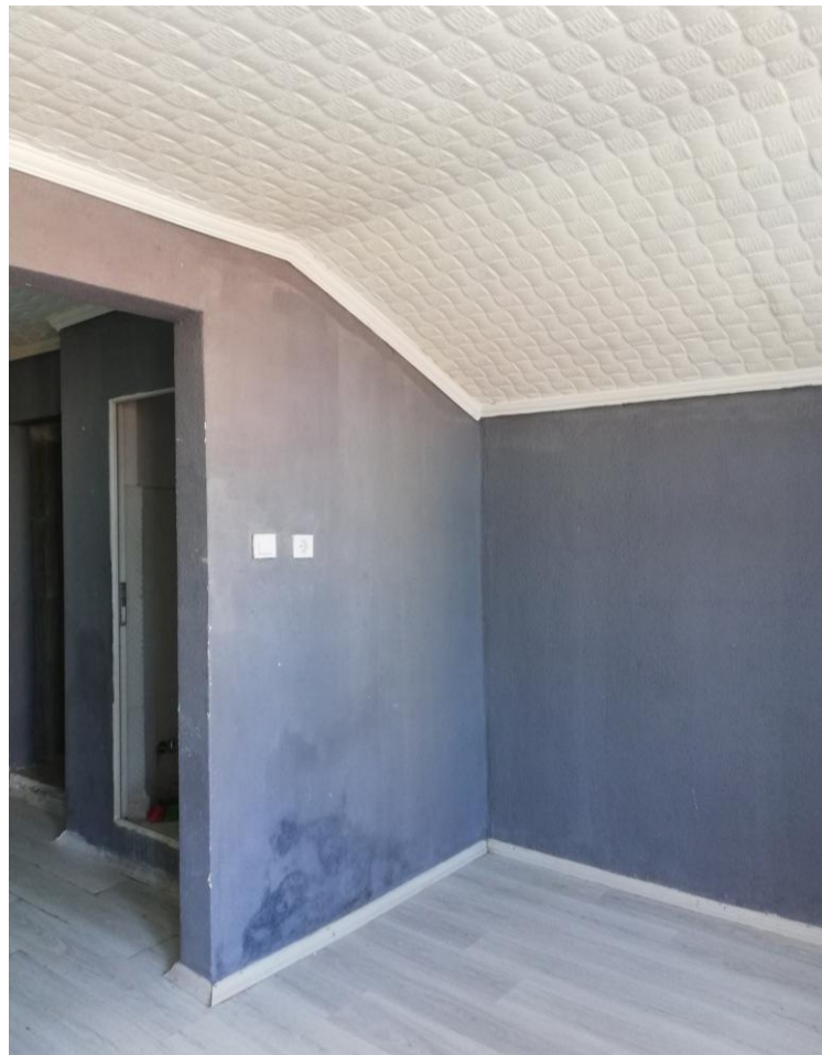
Figure 3.43. Moisture staining on fourth floor of Building C (Author, 2022)
