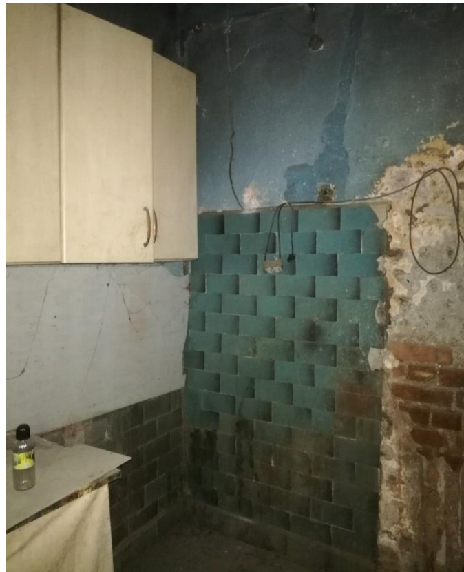
Figure 3.38. Deteriorations due to humidity on wall (Author, 2022)
