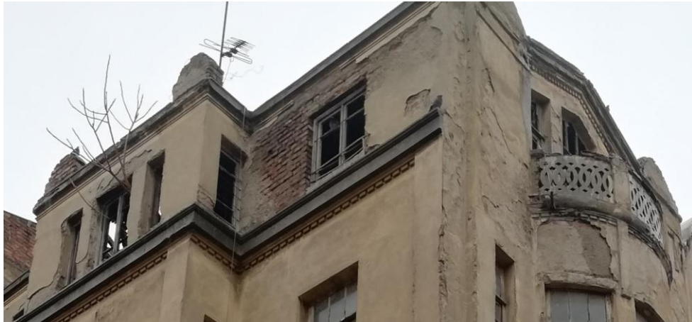
Figure 3.48. Plaster and paint detachment on the façade, Building D (Author, 2021)
