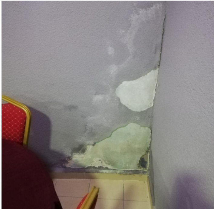
Figure 3.44. Loss of paint due to plumbing leak in basement, Building C (Author, 2022)
