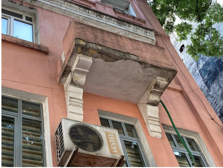
Figure 3.29. Anafartalar Street façade detaching of plaster (Author, 2021)
