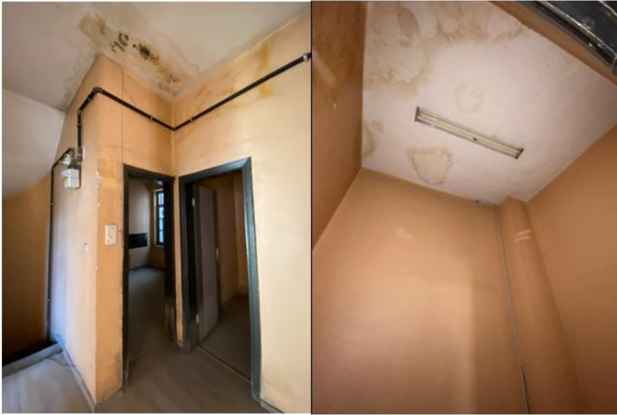
Figure 3.30. Building A staining due to humidity, Third Floor (Author, 2021)
