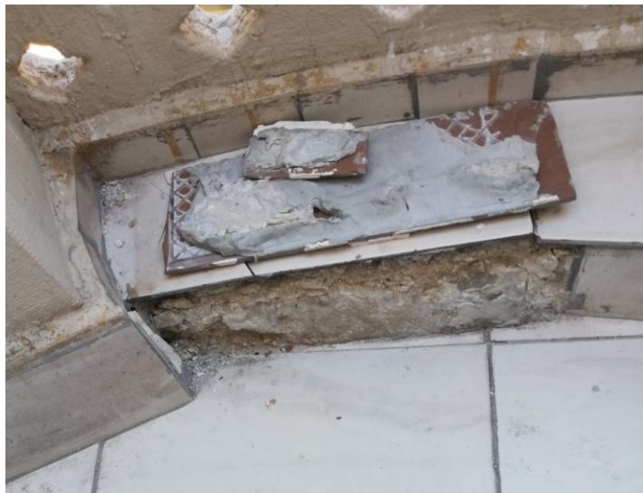
Figure 3.45. Deterioration of ceramics on the balcony, Building C (Author, 2022)
