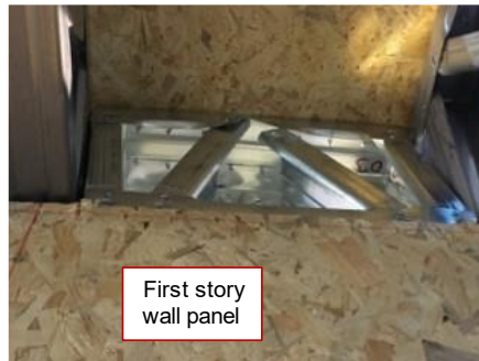
Figure 8.9 Failures observed in specimen WA-3
