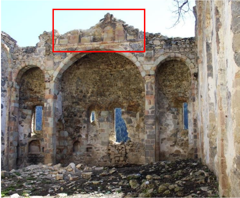
Figure 3.38: St. Christopher Church, the remaining parts of the decorative blind arcades
