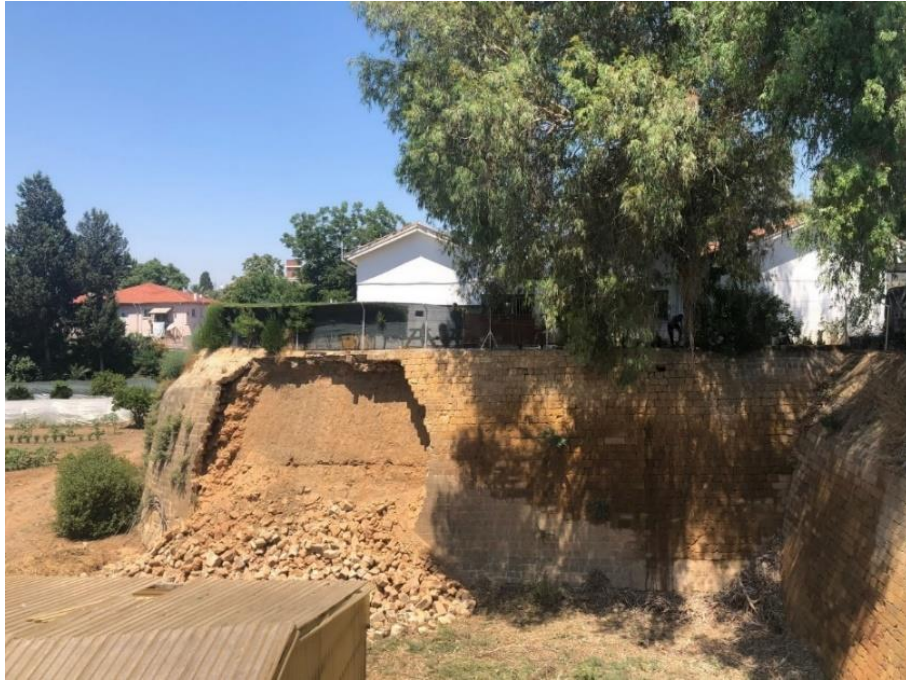
Figure 3.47a. Quirini Bastion of the Nicosia Fortifications in the northern part of Nicosia collapsed in 2019. (E. Reis archive 2019)
