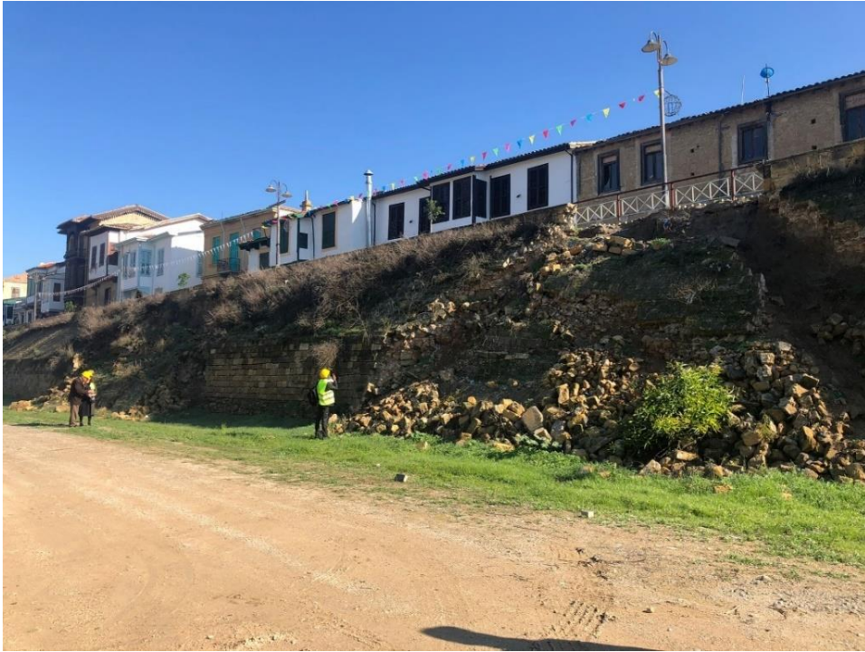
Figure 3.48a. Collapsed fortification walls of Zahra Street which are in Buffer Zone (E. Reis archive 2019)
