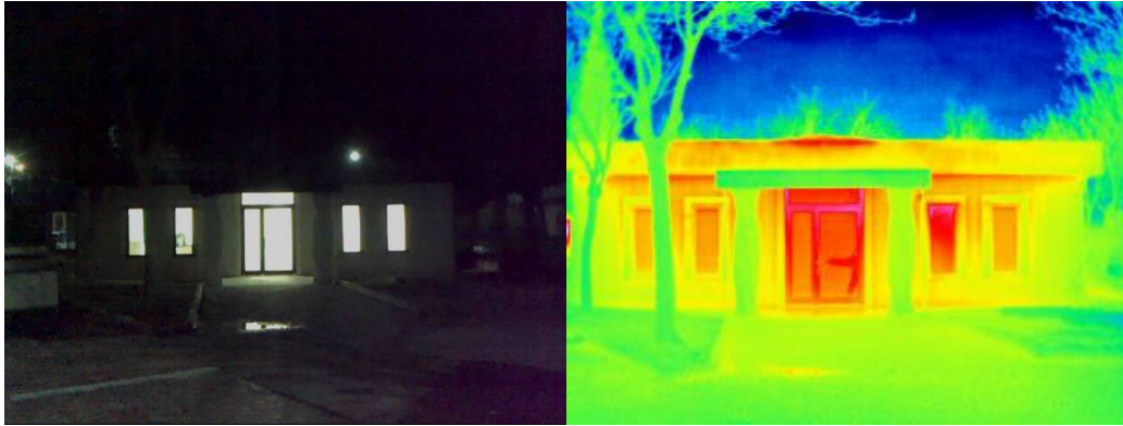
Figure 5.1. The thermal imaging completed between 2-5 am to minimize the convective heat loss
