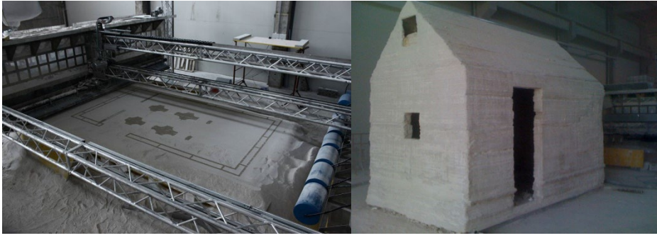
Figure 2.5. The production and final version of a structure printed on a D-Shape printer (D-Shape, 2015)
