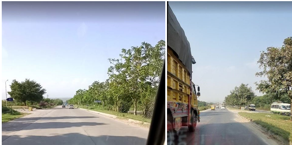
Figure 5.4. Absence of sidewalk outside Institute of Space and Technology, Islamabad. Source: Author
