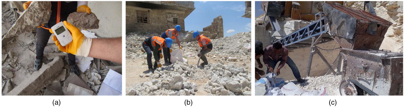
Fig. 3. Collection procedure for the RCA: (a) radiation measurements; (b) coning and quartering sampling method; and (c) crushing of concrete rubble with jaw crusher.
