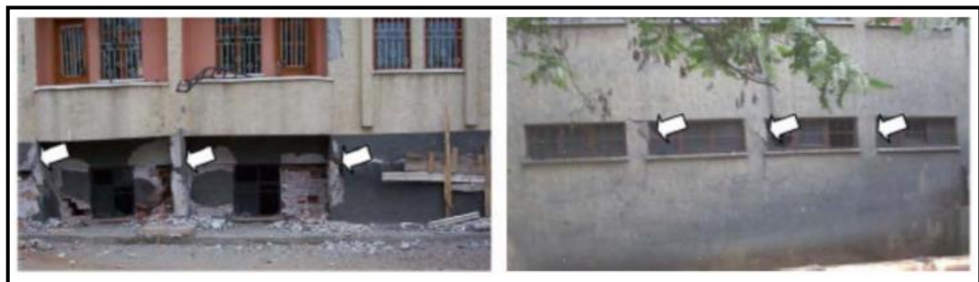
Figure 3.26: Damaged Building due to Short Column Effect
