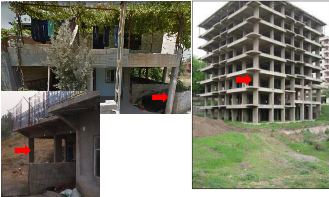
Figure 4.49: Insufficient Column Cross-Sectional Area
