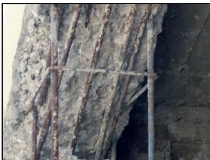
Figure 4.55: Open Reinforcements and Corroded Concrete
