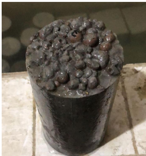
Figure 4.11 Segregation in Mix #3
