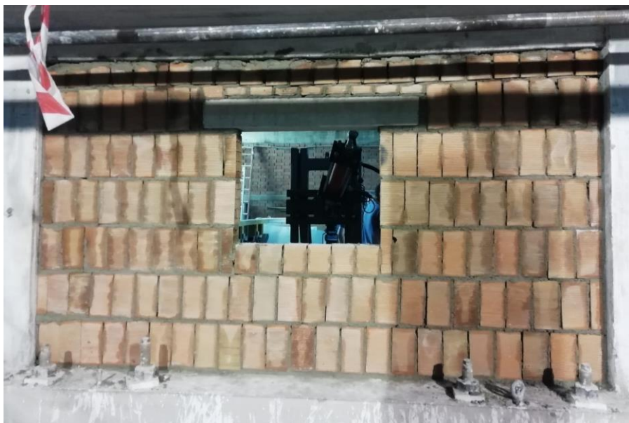
Figure 2.19. Built WBVW Without Plaster on it
