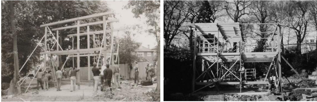
Figure 9: Users' participation in the building process and the construction of a dwelling unit following the Segal Method. Left image source: Kate Luxton, "Walter Segal Exhibition," Charlie Luxton Design, January 21, 2016, https://charlieluxtondesign.com/walter-segal-exhibition/ . Right image source: "Walter's Way: The Self-Build Revolution," ArchDaily, January 8, 2016, https://www.archdaily.com/780083/walters-way-the-self-build-revolution .
