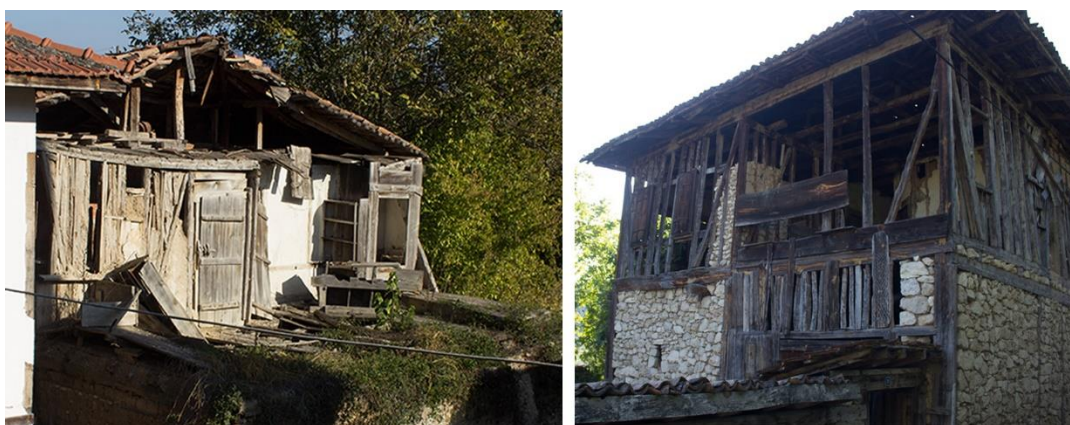
Figure 4.16. Hacilarobası, examples of buildings with severe structural problems
