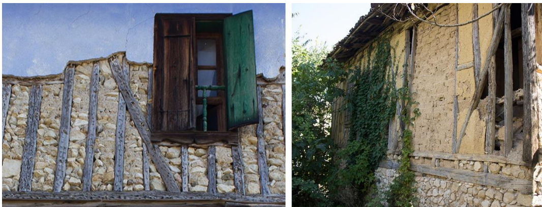
Figure 4.15. Hacilarobası, examples of deterioration on the facades
