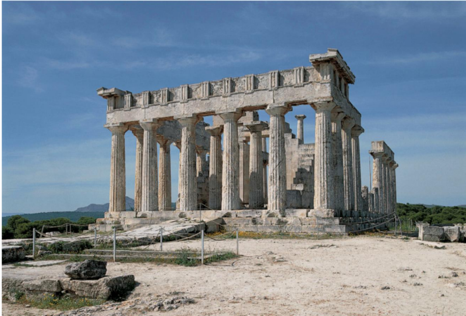
Figure 2.1: Temple of Aphaia in Aegina, Greece which has been standing in a high seismicity region for more than 2500 years[1]
