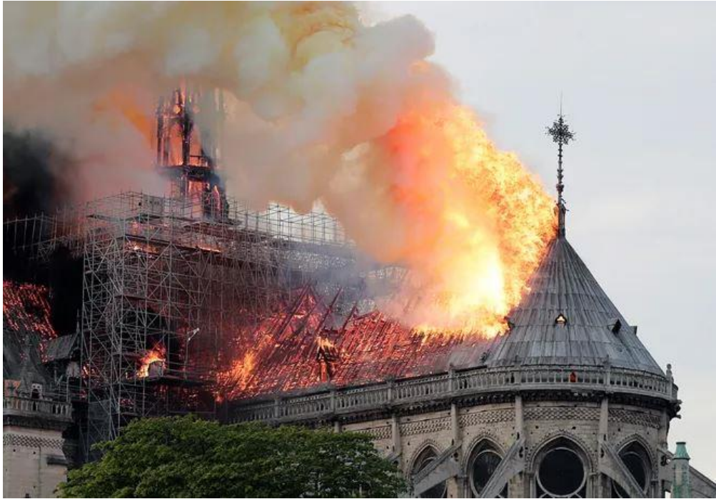
Figure 6.15. Notre-Dame' roof burning during the fire of April 15, 2019. (Source: https://www.usatoday.com/story/opinion/2019/04/16/notre-dame-cathedral-paris-fire-history-macron-column/3482618002/ )
