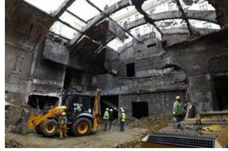
Figure 189 Construction works inside the building of the Emek movie theatre. (Source: Megaİstanbul, 2018)
