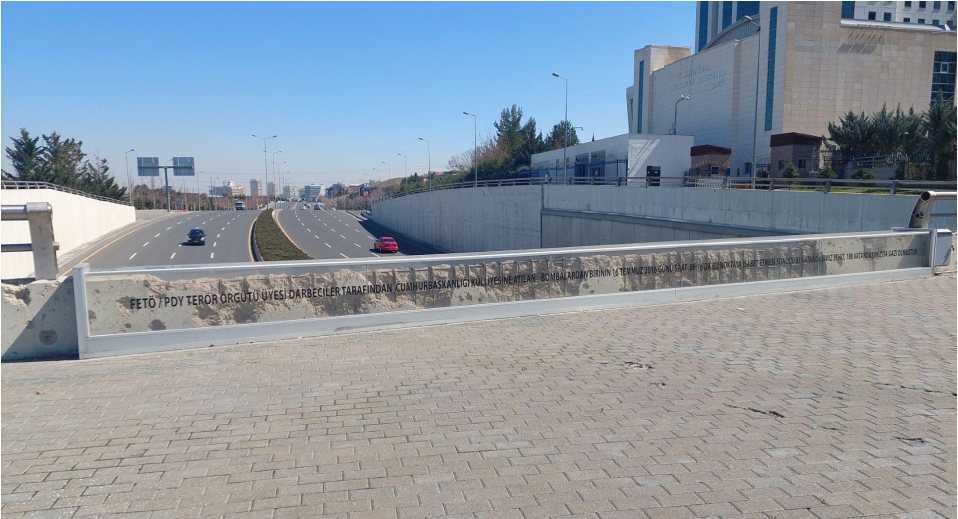
Figure 2. Exhibited parts of the Gendarmerie Underpass damaged as a result of gunfire from the air
