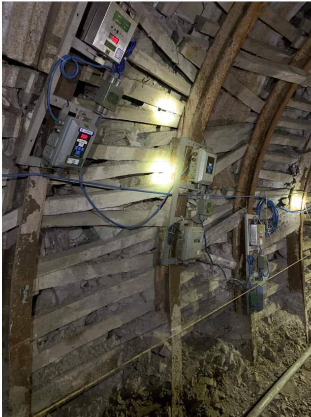
Figure 7: The measuring sensors of the dangerous gases inside the furnace.
