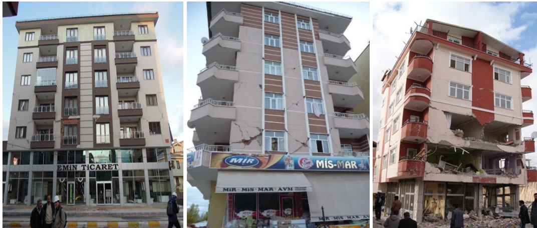
a) Light infill damage b) Moderate infill damage c) Heavy infill damage
