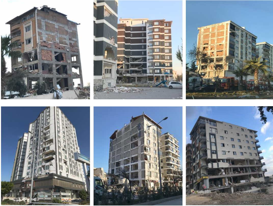
Figure 1.7. OOP failure of infills, 2023 Kahramanmaraş EQ ( M_w=7.7 )
