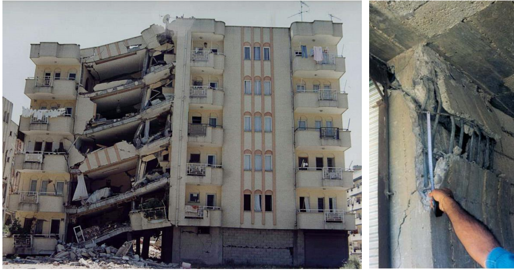
Figure 1.6. Different damages on identical blocks, 1998 Ceyhan EQ ( M_w=6.2 )
