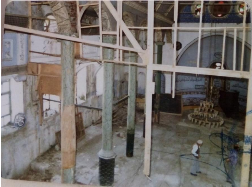
Figure 3.30. Aydinpinar, Hagios Ioannes, naos as seen from the gallery floor (BKVKBK Archive, 1986)
