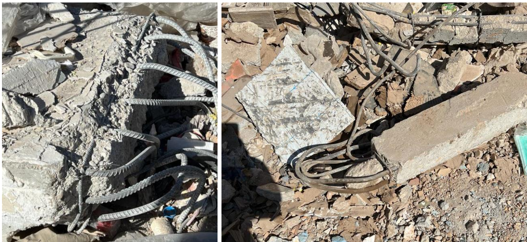
Figure 2. Deformed and plain reinforcement details from Antakya, Hatay
