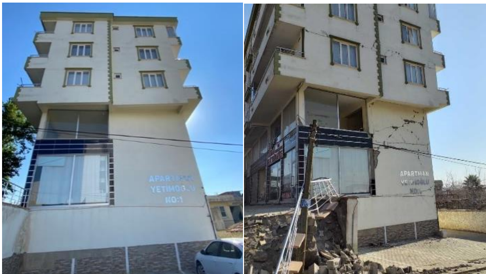
Figure 50. An example building in Turkoglu, before and after the earthquake
