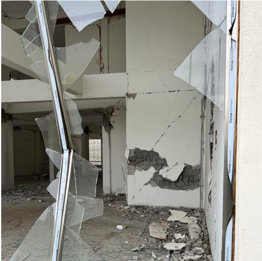
Figure 1. Failure of a shear wall from Kahramanmaraş
