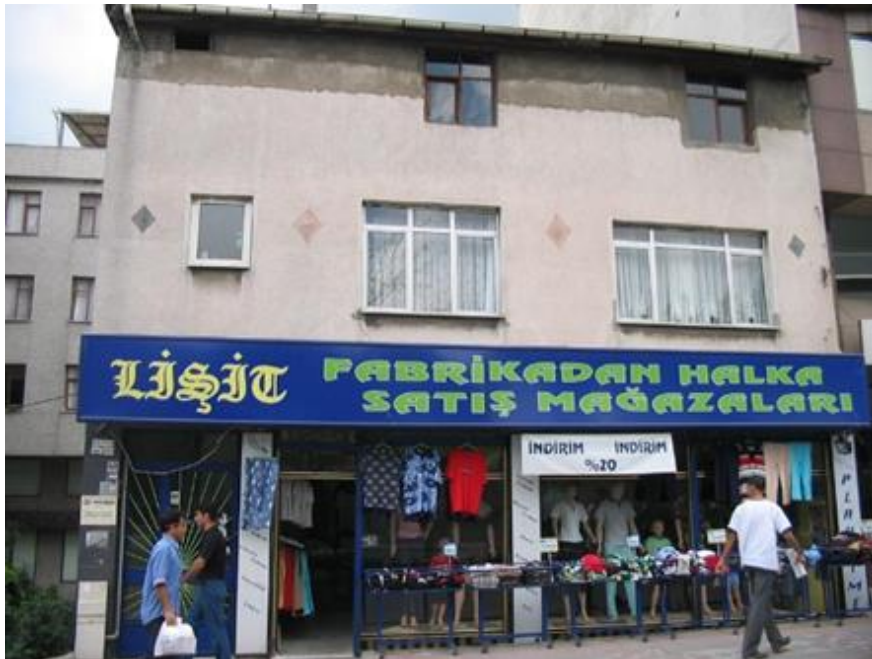
Figure 4. A real-life example of a building with a soft ground story
