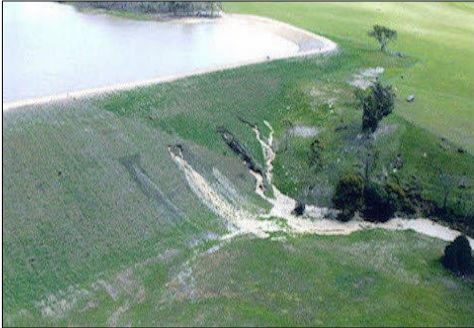
Figure 1.1 An aerial photo from an earthen dam subject to excessive internal erosion. The location is not known (Belcher et al., 2016).
