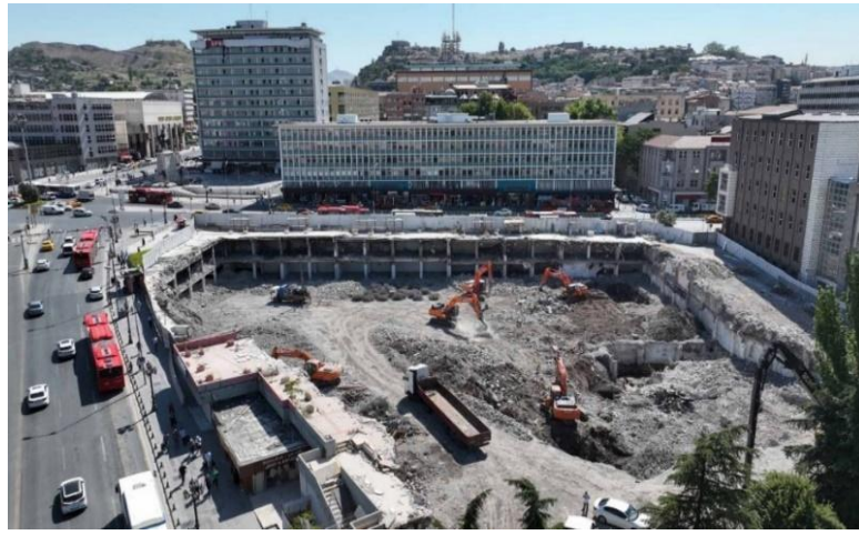
Figure 47: An aerial view of the area after the demolition of the 100. Yıl Bazaar. Source: AMM, 2023e.
