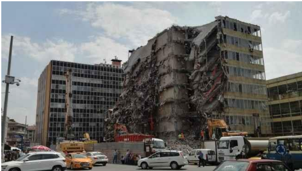
Figure 40: An image from the demolition of the office block of Anafartalar Bazaar. Source: Kaplan, 2022.
