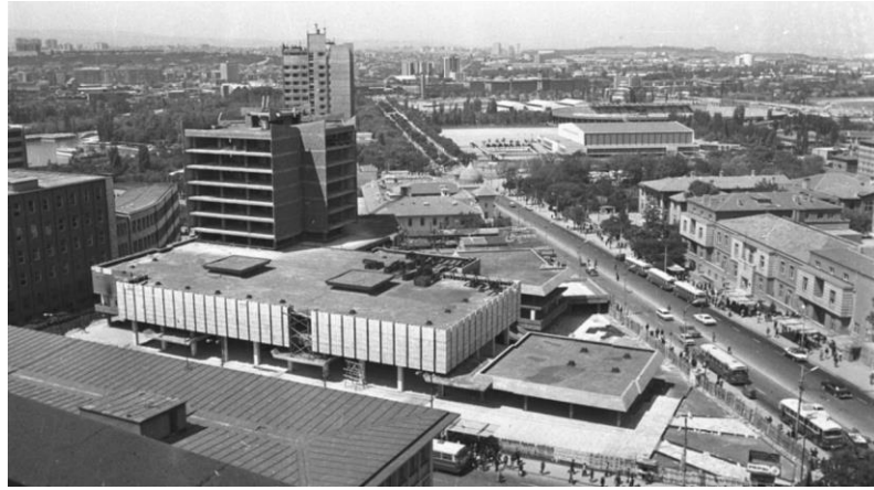
Figure 27: A view of the 100. Yıl Bazaar under construction. Source: Retrieved from TRT Archive by Kızıl, 2023, p. 67.
