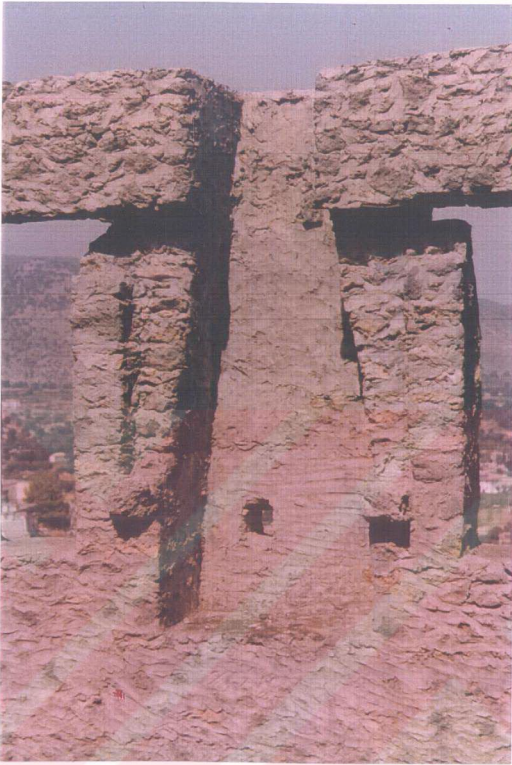
Figure 3.37 : Unfinished Construction of Wall Type Fire Place
