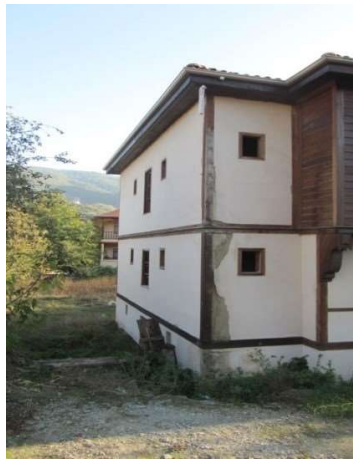
Figure 4.62. Current view of east side facade that indicate the F.AD1 and F.AD2 (Author, 2013)
