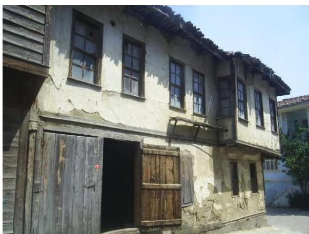
Figure 3.29. Pre intervention east facade view of Abdi İbrahim house (taken from the Taraklı Municipality, 2013)
