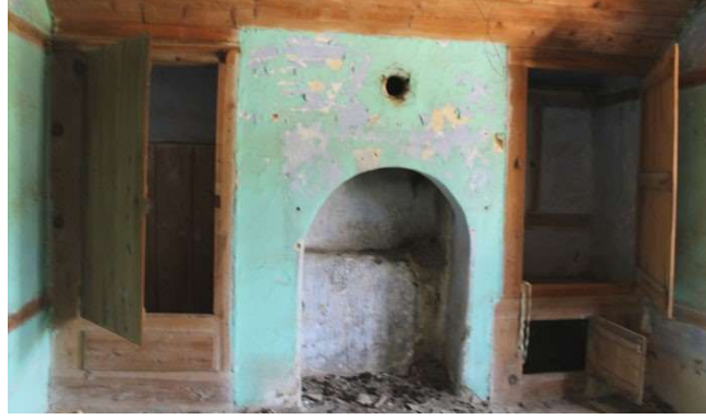
Figure 2.20. Gusülhane (at left side of fireplace) , fireplace and closet (at right side of fireplace) view of the room, Haşmet Doğru house (Author, 2016)
