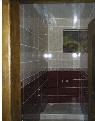
Figure 4.77. Alterations of FPOI03 during the hotel transformation of Çakırlar House (taken from the Taraklı Municipality, 2013)
