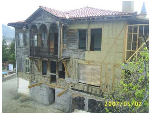
Figure 3.6. Pre-intervention view of Kadirler house, north facade (taken from the Taraklı Municipality, 2013)
