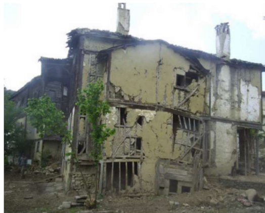
Figure 4.63. Pre-intervention view of east side facade that indicate the F.AD1 and F.AD2 (Özkan, 2008, p.123)
