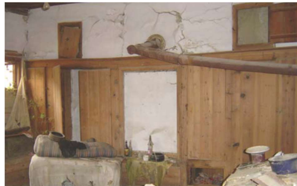
Figure 4.68. Pre-intervention view of closets at second floor of the house (Özkan, 2008, p.111)
