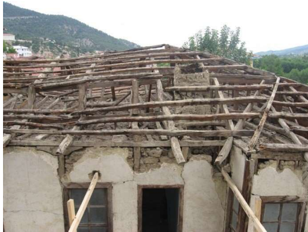
Figure 2.11. Wooden structure of the roof of Abdi İbrahim house before hotel transformation (taken from the Taraklı Municipality, 2013)
