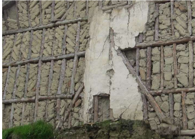
Figure 2.13. Mudbrick detail as a construction material from unnamed house in Taraklı (Author, 2016)
