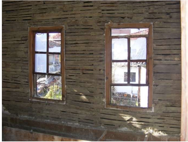
Figure 2.15. Bağdadi system in unnamed house in taraklı (taken from the Taraklı Municipality, 2013)
