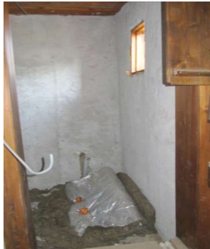
Figure 3.70. Wet space addition inside the closets at rooms of mezzanine floor (Author, 2013)
