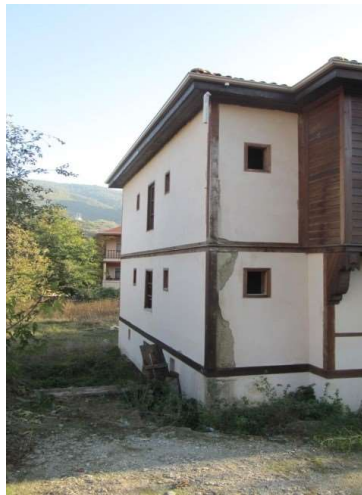
Figure 4.55. Current view of east side facade that indicate the G.AD1 and G.A1 (Author, 2013)
