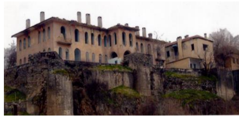
Figure 41. The east facade of Government House from the Tigris Valley before restoration, n.d.
