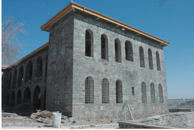
Figure 43. The south facade of the Government House, during the restoration. (Gökhan Baydaş, 2007, p. 352.)
