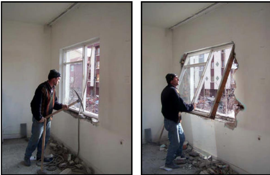
Figure 2.4. Damage from the dismantling process of a window (Çakıcı, 2005).
