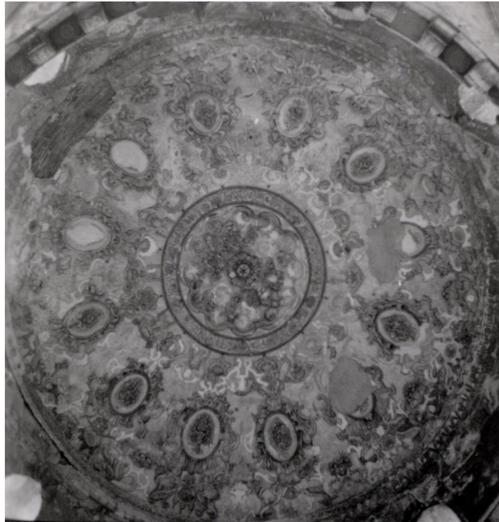
Figure 19. Aydın Cihanzade Mosque's dome before the restoration (SALT Archives, Ali Sami Ülgen Photograph Collection)
