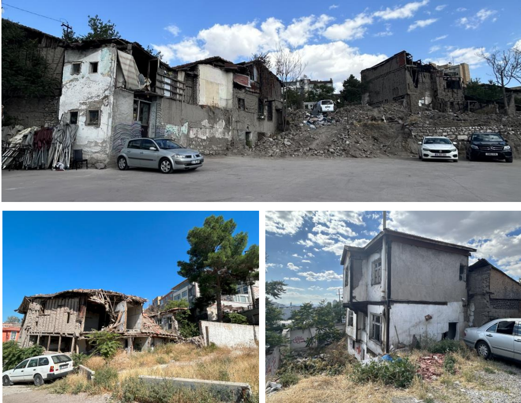
Figure 3.33. Traditional buildings that have major structural problems and partially collapsed (Author, 2024)
