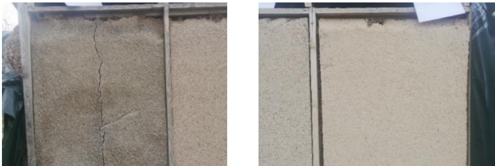
Figure 3-3. (Left) Crack on the surface of panel A1(KeSdMo)(Right), Surface of panel C3(KeSdFb-2).
