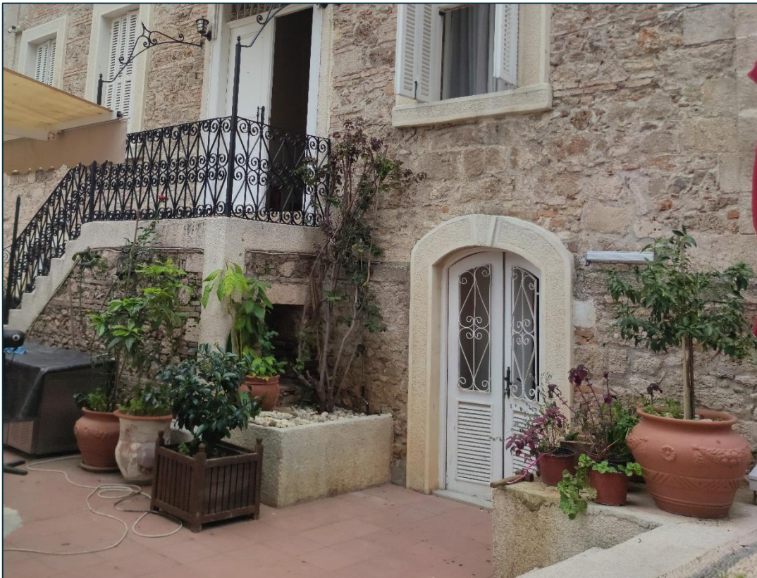
Figure 3.91. Added doorway within the previously closed masonry wall in Building B. Taken by the Author.
