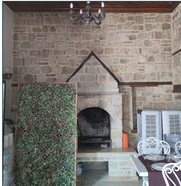
Figure 3.67. New stone and brick composite wall replacing the original stone masonry one. Taken by the Author.
