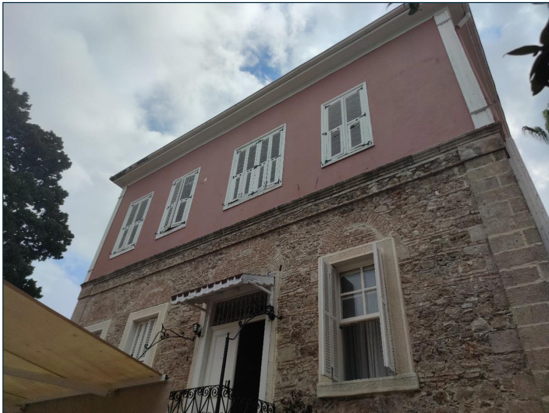
Figure 3.43. Photograph of the courtyard (Northwest) elevation of Building B. Taken by the Author.
