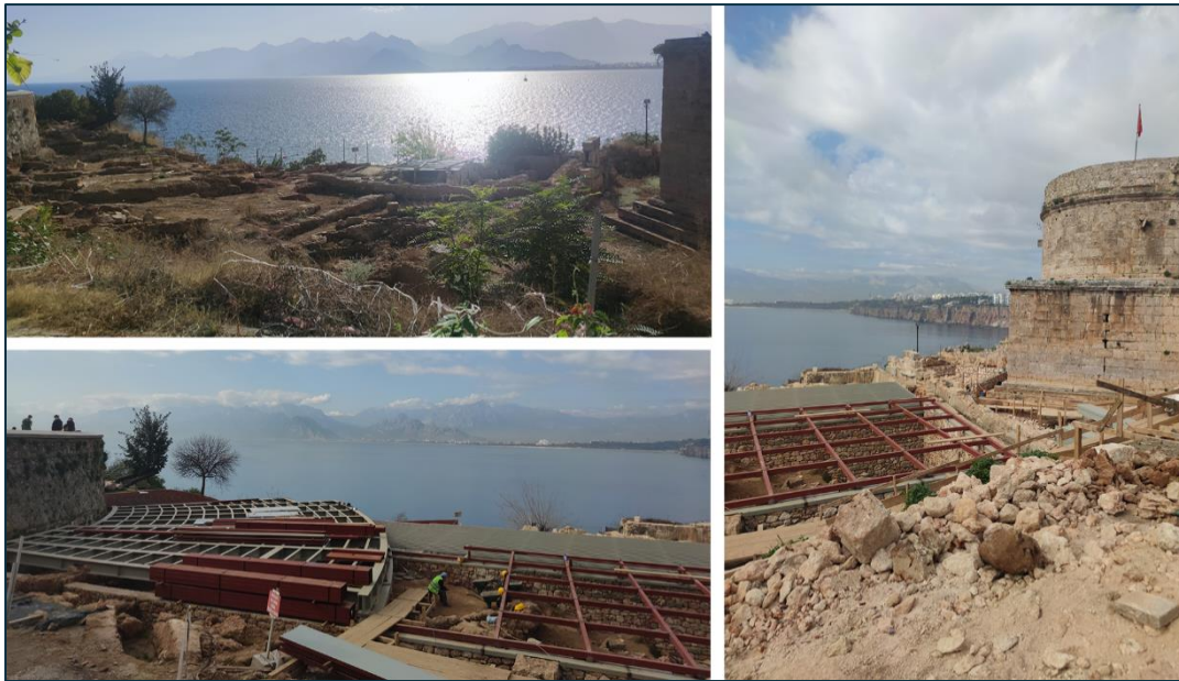
Figure 3.22. The before and during of the Conservation and Development Project of Hıdırlık Tower. Taken by the Author on 23/09/2023 and 07/02/2024.
