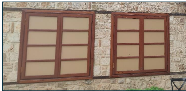
Figure 3.77. Enlarged opening with new materials and technique windows. Taken by the Author.
