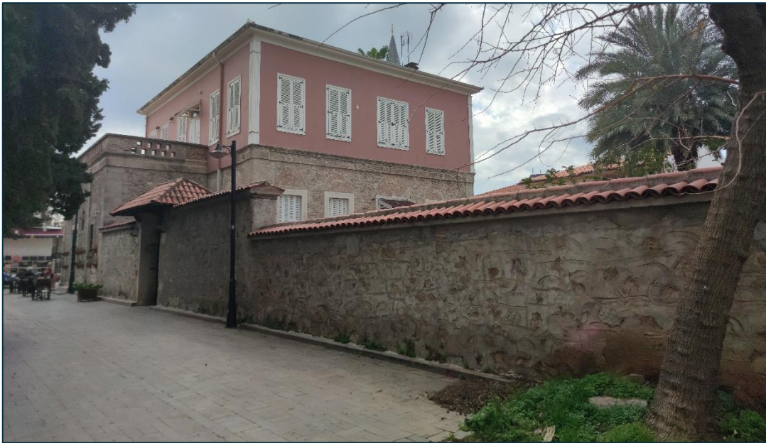
Figure 3.32. Photograph of the lot wall of Building B. Taken by the Author.
