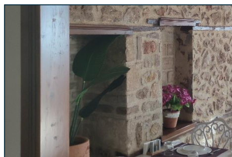
Figure 3.78. Maintained and cleaned niche (right) and dismantled then rebuilt niche with new interior materials (left). Taken by the Author.
