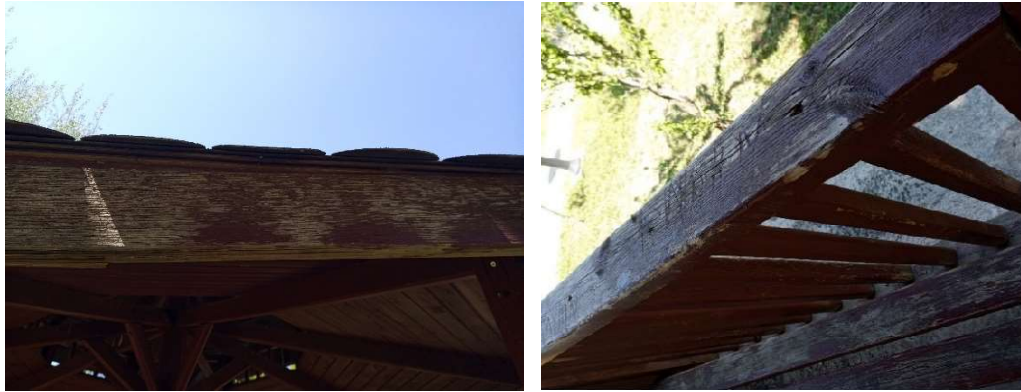
Figure 4.14: Signs of weathering on the wooden gazebo in Area 4
