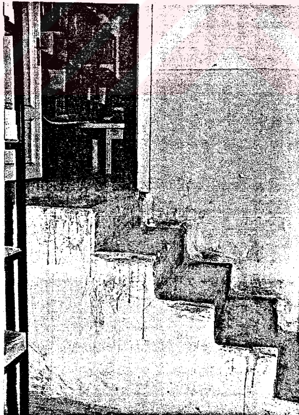
Photo.47 The Central building - basement floor - SW of the second storage room on the SW (1987)
