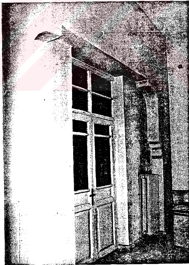
Photo.27 NW wing - ground floor - Bursa arches in the room on the NW (1987)
