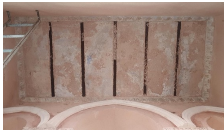
Figure 31. The ceiling of entrance hall of the tomb of Grand Vizier Ahmet Cevad Pasha and the iron profiles (taken by the author in 2021)
