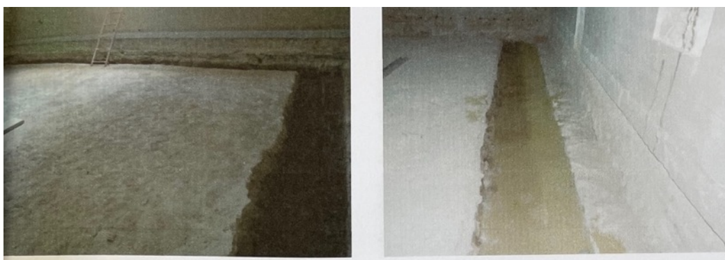
Figure 192. The photographs of the excavation along load bearing walls the ground level of 3 rd Construction Phase of IAM (source: IDSM Archive)
