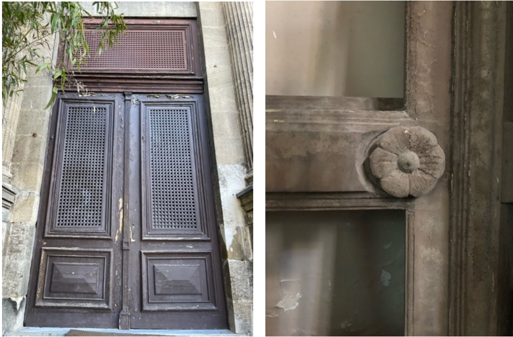
Figure 155. (Left) Exterior wooden door (Right) interior wooden door detail (taken by the author)
