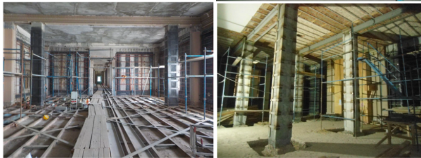
Figure 129. Photographs that were taken during Reinforcement and restoration works on ground floor, Left: Hall 28, Right: Hall 19 (source: IDSM Archive)
