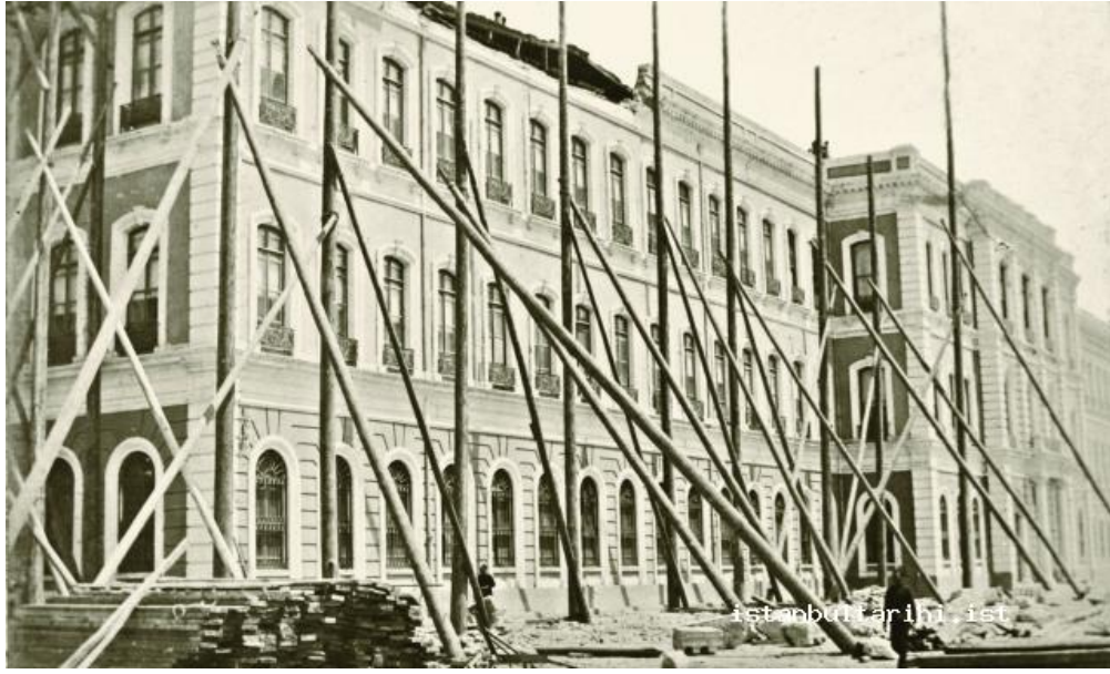
Figure 49. The repair works in the Daire-i Umur-i Askeriye building damaged in the earthquake (source: İstanbul Atatürk Kitaplığı, “İstanbulda Vuku Bulan Büyük Hareket-i Arz’a ait Albümler”, Nr.184/2- https://istanbultarihi.ist/27-bir-sehir-manzarasi-istanbulun-tarihinde-depremler )
