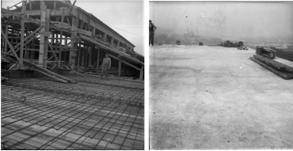
Figure 113. The photographs that were taken during the Conversion of the Roof of IAM from Timber to Concrete (1948-1956)
