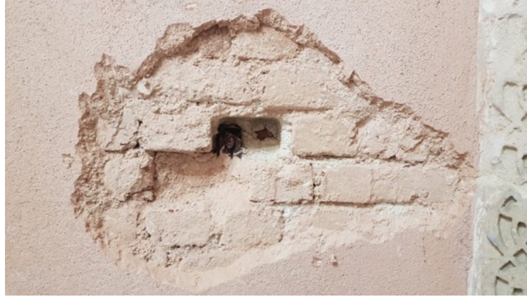
Figure 29. The clamp detail from the inner section of wall of the tomb of Grand Vizier Ahmet Cevad Pasa (taken by the author in 2021)
