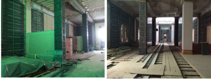
Figure 128. Photographs that were taken during Reinforcement and restoration works on columns and walls, Left: Hall 13-14-15 Right: Hall 25 (source: IDSM Archive)
