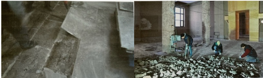
Figure 190. The removal of marble and cement layer from the ground floor of 3 rd phase of IAM building.
