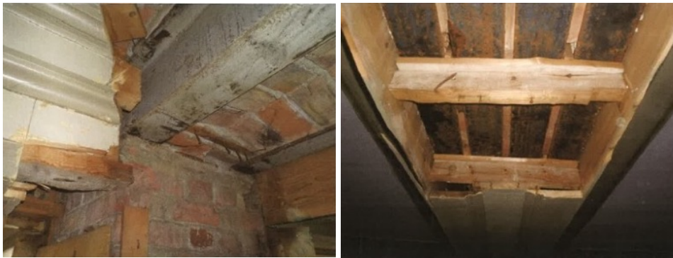
Figure 245. (Left) The photograph of AA section of Hall 22 jack arched flooring detail (Right) The photograph of BB section of Hall 21 jack arched flooring detail ( Güryapı İnşaat Construction site report, November 2012, drawn by Rabia Şengün, IDSMArchive).
