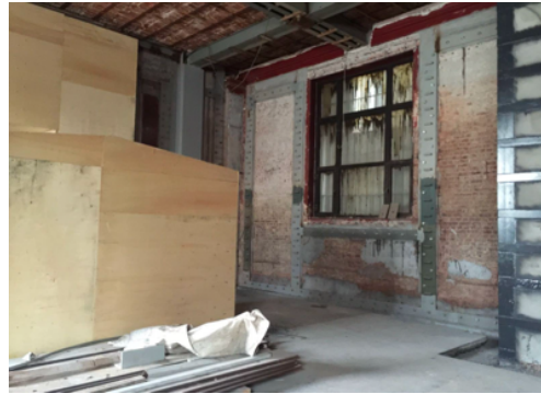
Figure 276. The brick masonry wall construction Techniques of 1 st Phase of IAM (1887-1891) (taken by the author)
