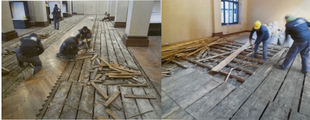
Figure 225. The removal of wooden parquet from first floor of 3 rd Construction Phase of IAM (source: Güryapı İnşaat Company , IDSMArchive)
