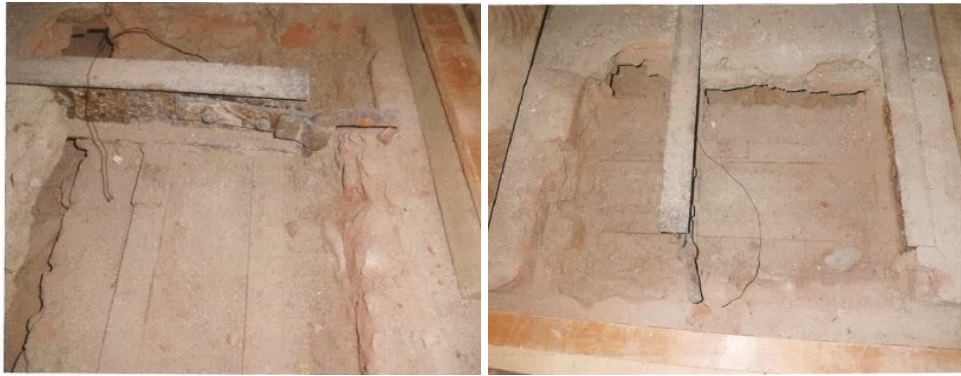
Figure 247. The Photographs of AA section drawing of Hall 21 jack arched flooring details ( Güryapı İnşaat Construction site report, November 2012, IDSM Archive).
