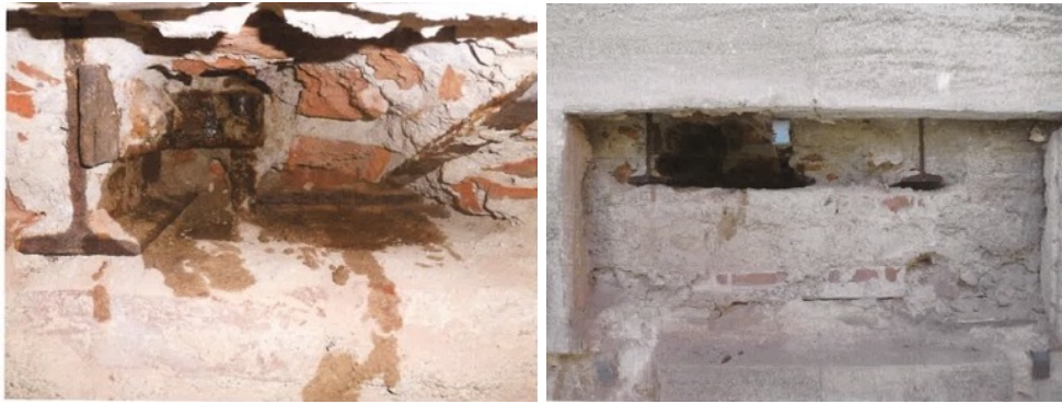
Figure 248. The Photographs of BB section drawing of Hall 21 jack arched flooring details ( Güryapı İnşaat Construction site report, November 2012, IDSM Archive)
