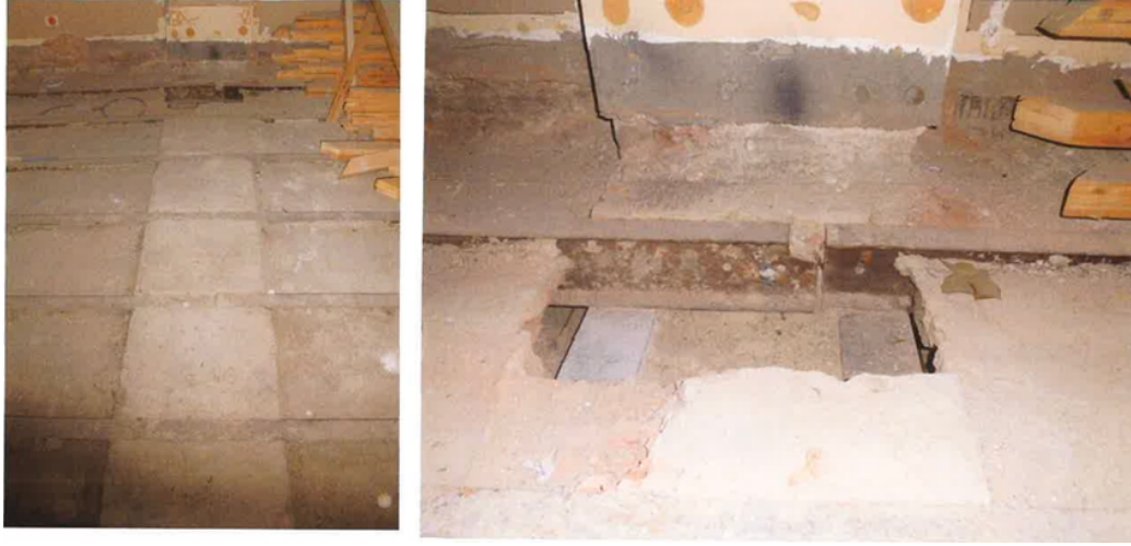
Figure 254. The Photographs of BB section drawing of Hall 23 jack arched flooring details ( Güryapı İnşaat Construction site report, November 2012, IDSM Archive)
