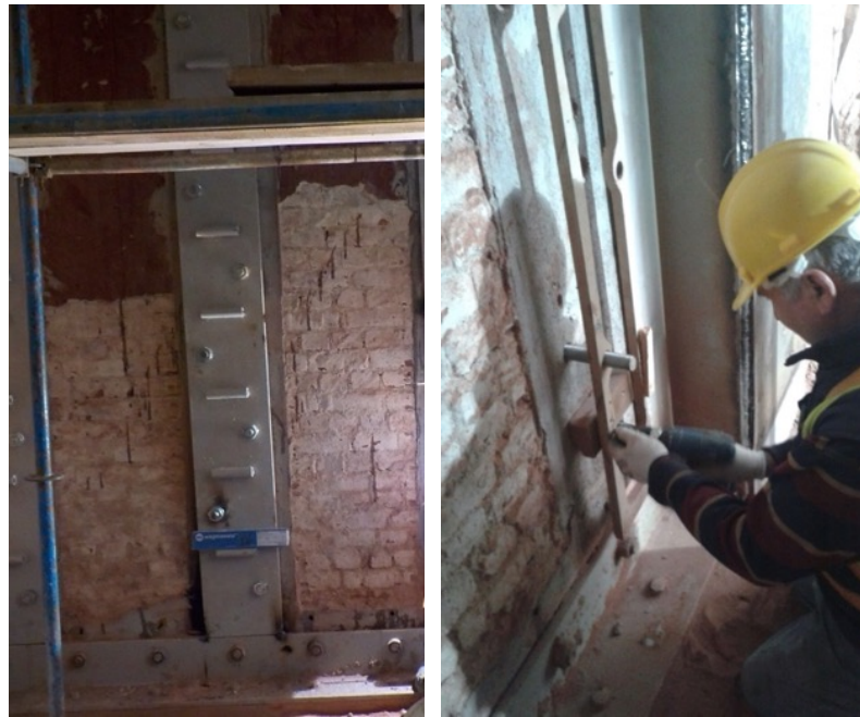
Figure 207. The photo showing brick masonry walls of 1 st phase of IAM taken during strengthening work in between 2011-2017 (source: Güryapı İnşaat , IDSM Archive)
