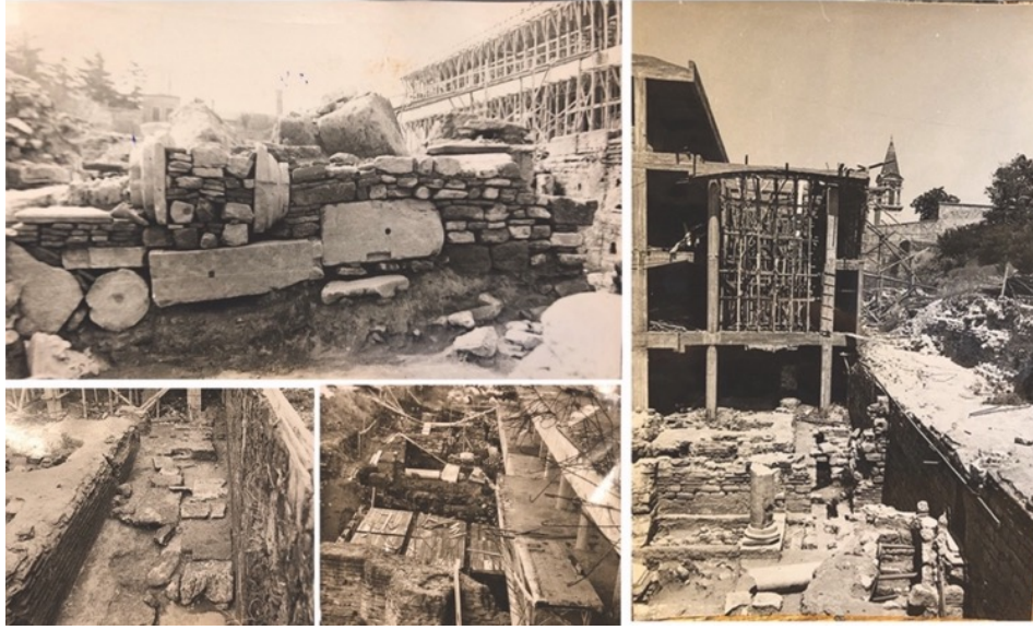
Figure 73. The photos of the foundation excavation during the construction of the Additional Building (source: The Personal Achive of Nezhir Fıratlı, IAM-Archive) (Üstođlu Coşkun & Şahin Güçhan, 2024)
