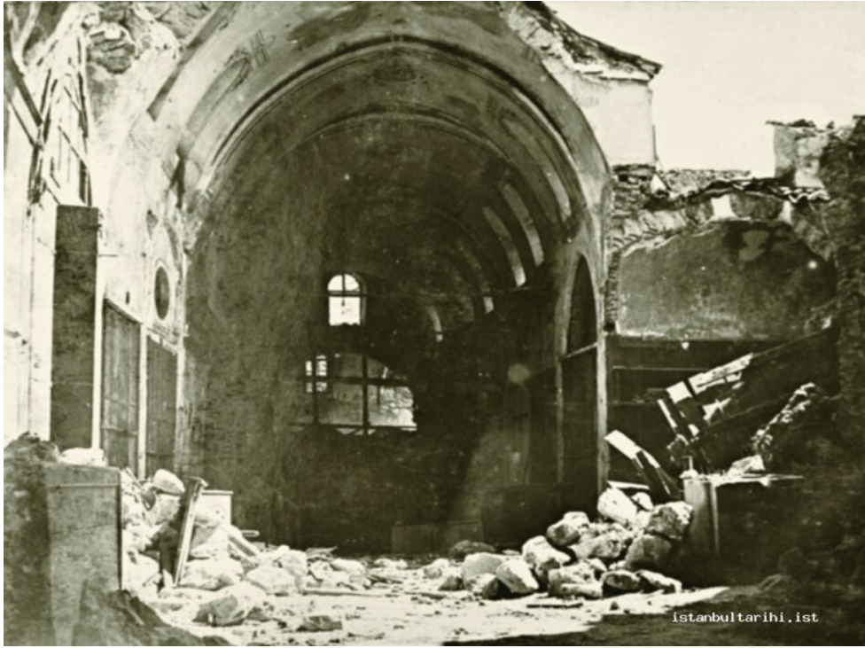
Figure 44. The 1894 earthquake and the damage it caused in Istanbul (source: İstanbul Atatürk Kitaplığı)
