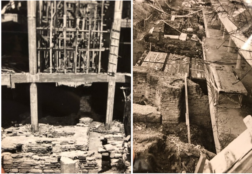
Figure 121. The Photos of the construction of Additional Building in the excavated area (source: The Personal Achieve of Nezhir Fıratlı, IAM Archive)
