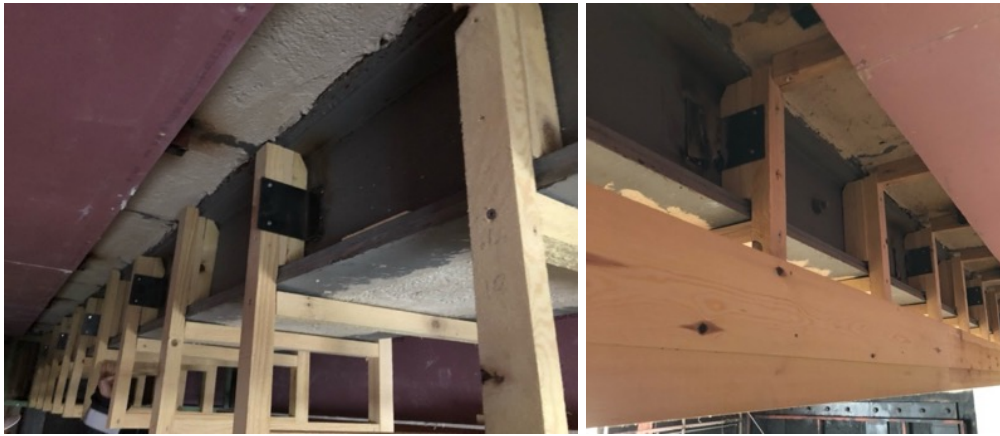
Figure 268. Construction of new wooden cornices to the iron beams with traditional techniques with some metal addition (taken by the author in 2019)
