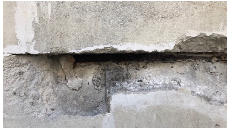
Figure 30. The clamp detail from the outer section of the wall of the tomb of Grand Vizier Ahmet Cevad Pasa (taken by the author in 2021)
