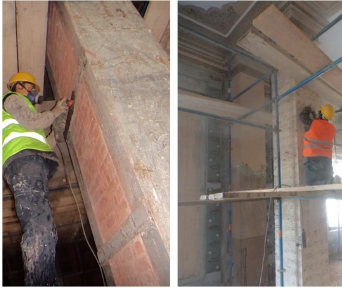
Figure 208. The photo showing brick masonry columns of 1 st phase of IAM taken during strengthening work in between 2011-2017, left ground floor right: 1 st floor (source: Güryapı İnşaat , IDSM Archive)
