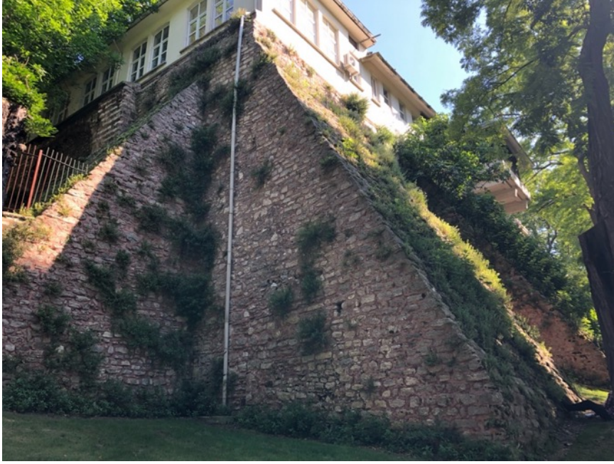
Figure 61. The buttresses under the Sanayi-i Nefise Mektebi (source: taken by the author in 2021)
