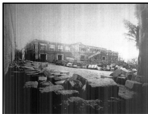
Figure 277. The stone masonry with brick lintel wall construction Techniques of 2 nd Phase of IAM (1899-1903) (source: Restitution Report prepared by Seçkin Mimari Hizmetleri, IDSM Archive)
