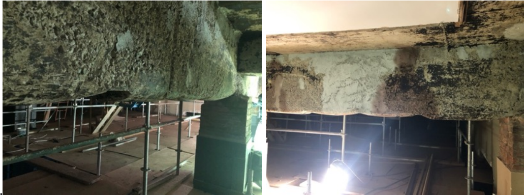
Figure 116. The reinforced concrete beams of 1 st floor of 3 rd Construction phase of IAM (source: taken by the author in 2018)
