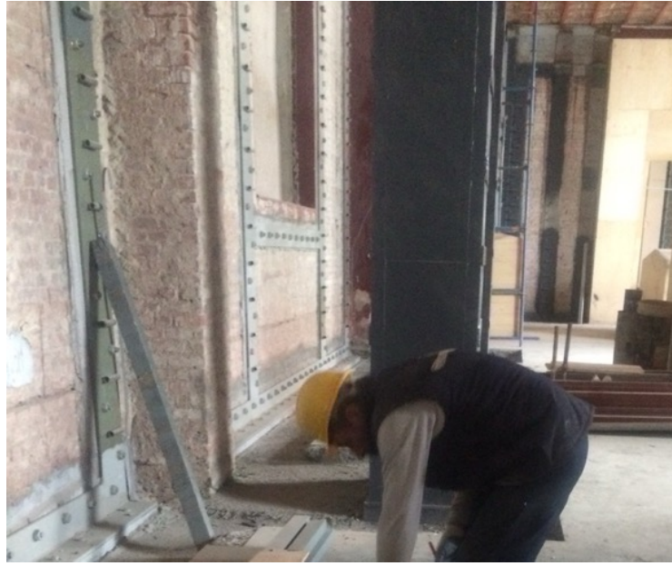
Figure 206. The photo showing brick masonry walls of 1 st phase of IAM taken during strengthening work in between 2011-2017 (source: Güryapı İnşaat Company, IDSM Archive)
