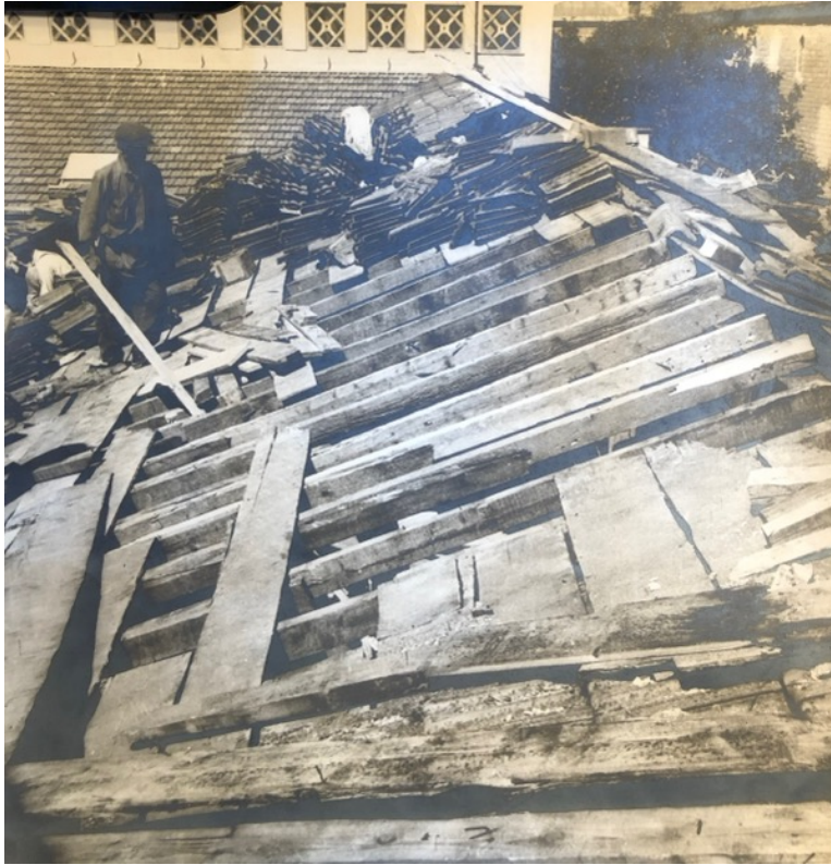
Figure 272. The old photograph showing the removal of timber roof (source: IAM Archive)
