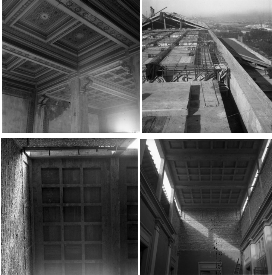
Figure 114. The conversion of roof floor and roof lanterns to reinforced concrete in 2 nd Construction phase of IAM (source: IAM-Photograph Archive)
