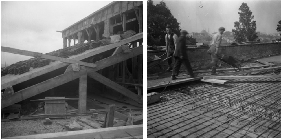
Figure 112. The photographs that were taken during the Conversion of the Roof of IAM from Timber to Concrete (1948-1956)
