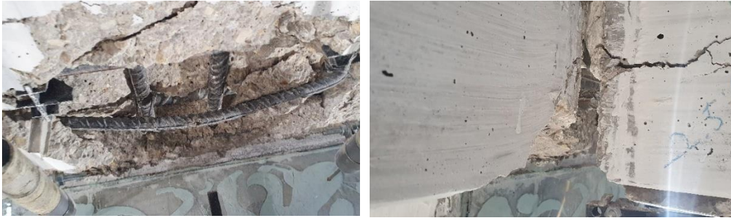
(a) Bar buckling
