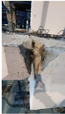
(a) Slab reinforcement rupture
