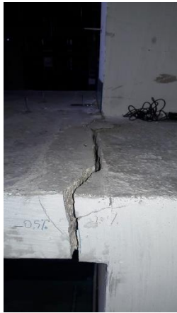
(a) Slab cracking
