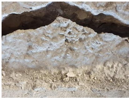
(a) Slab cracking
