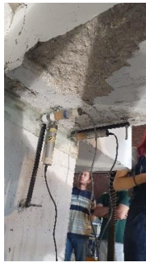
(b) Concrete cover spalling
