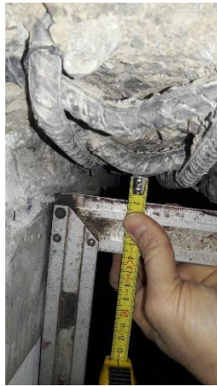
(b) Bar buckling
