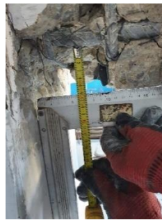
(b) Bar buckling
