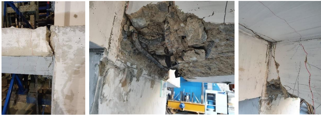
(a) Slab cracking
