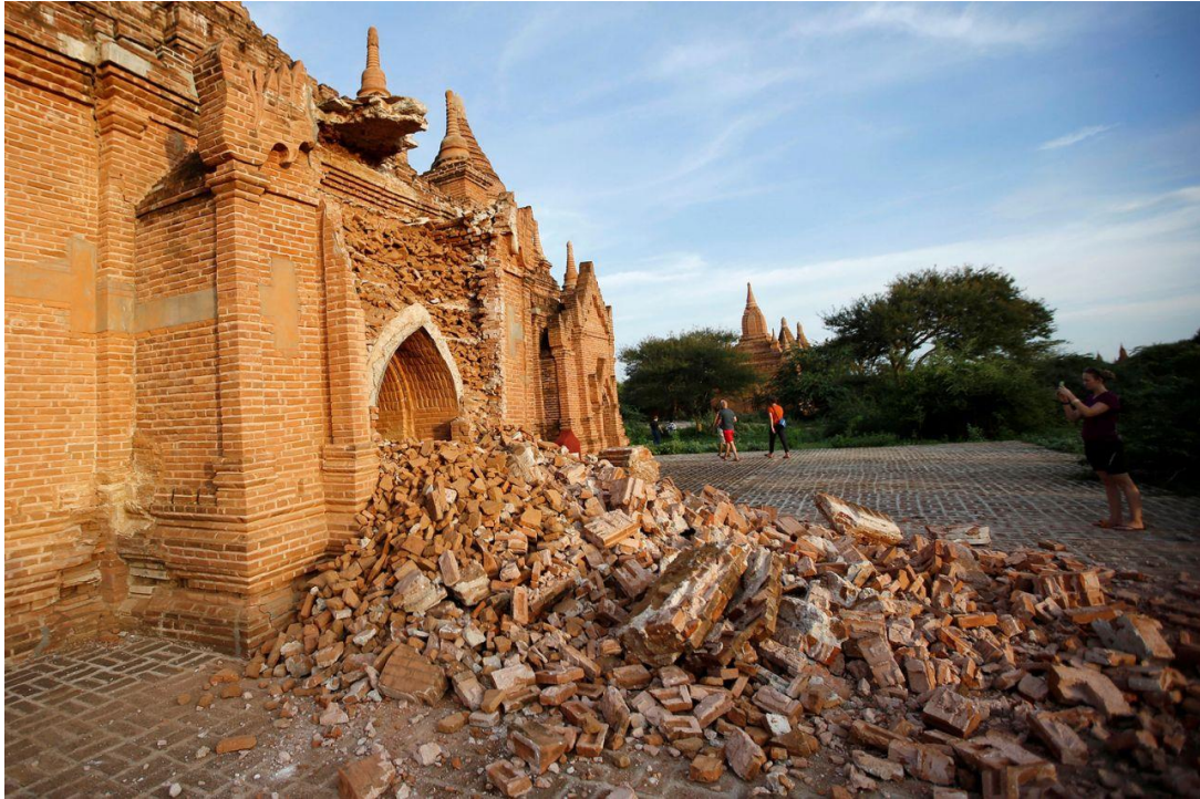
Figure 20. A Historic Buddhist Temple in Myanmar Following the 2016 Earthquake 59
