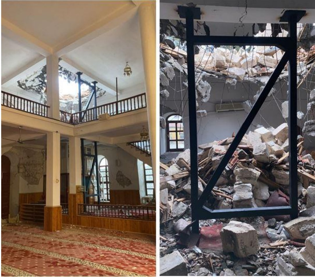
Figure 55. Structural Support Addition in Enver-ül Hamit Mosque in Osmaniye Province Following the Earthquake
