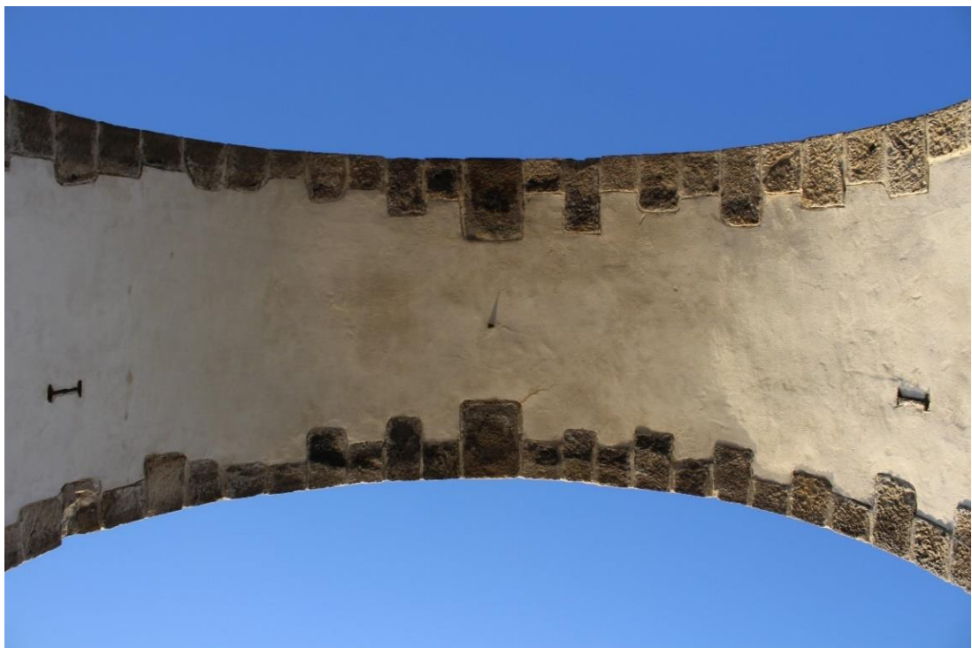
Figure 61: Şarjöman Rapid, overview (top), steel reinforcements in the arch and view from underneath (bottom), photos taken by the author
