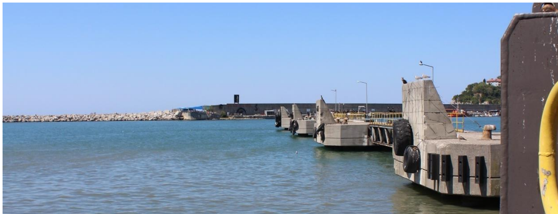
Figure 40: Train Ferry Dock overview (top), breasting dolphins (bottom), photographs taken by the author
