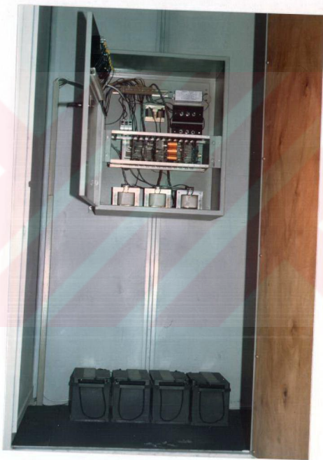
Figure 1.5 Controller and Batteries
