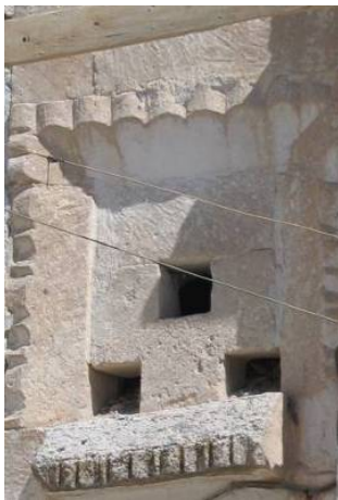
Figure 3.75 Birdholes on front facade of a house
