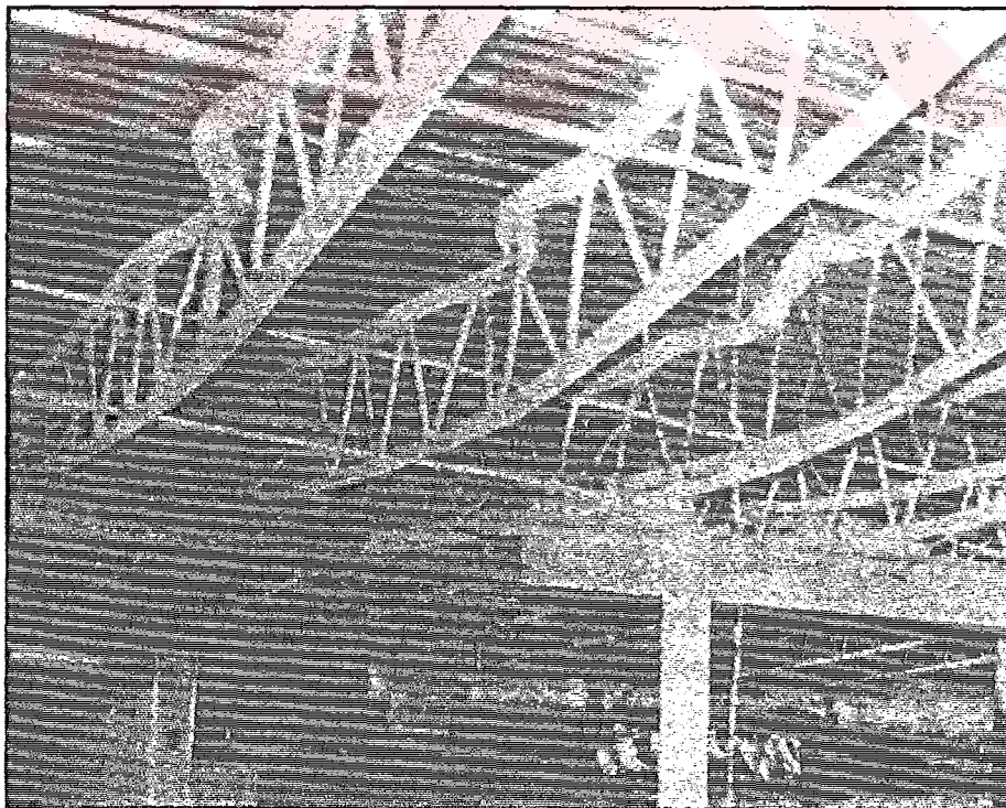
Figure 3.1 Typical fire damage to unprotected steel trusses in restrained conditions
