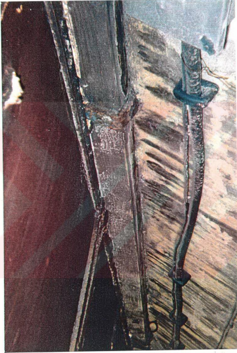
Figure 30- Metal awning in between two storeys on the S.W. facade facing courtyard
