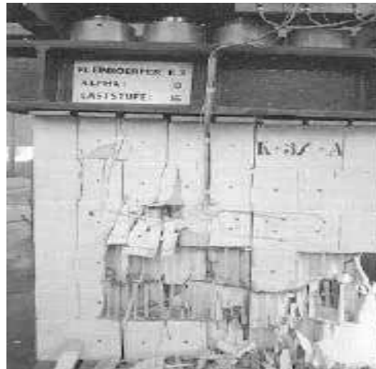
Figure 2.5. Compression failure of masonry units
