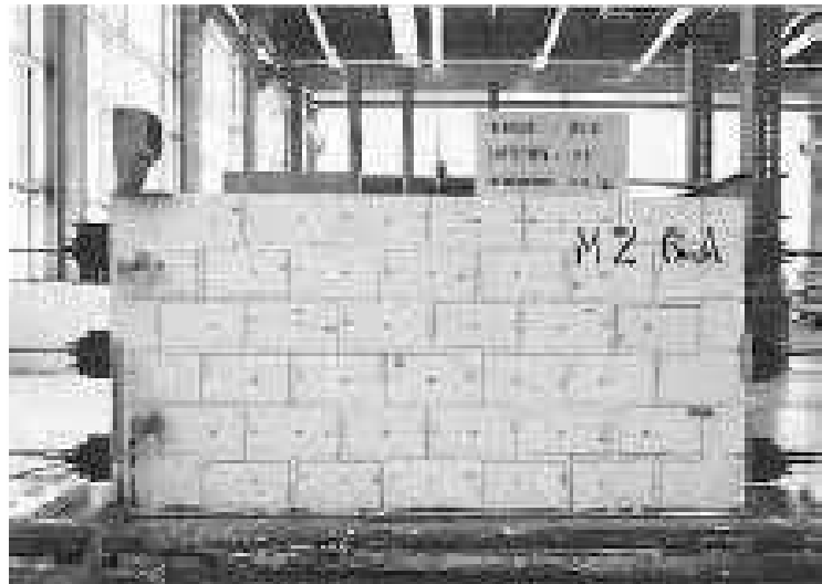
Figure 2.9. Tension failure along joints
