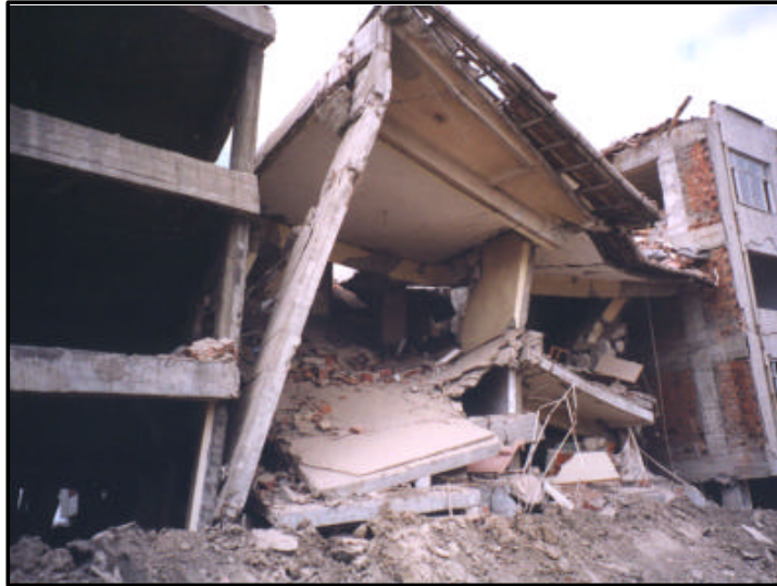
Figure 2.15: Failures due to irregularities of structural members
