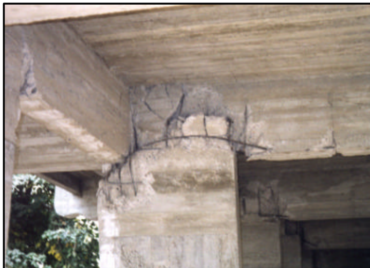
Figure 2.11: Buckling due to insufficient reinforcement
