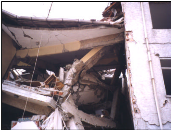
Figure 2.16: Failures due to irregularities of structural members
