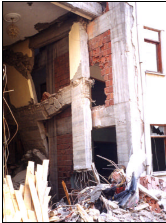
Figure 2.14: Failures due to irregularities of structural members
