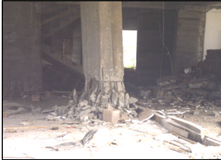
Figure 2.10: Buckling due to insufficient reinforcement
