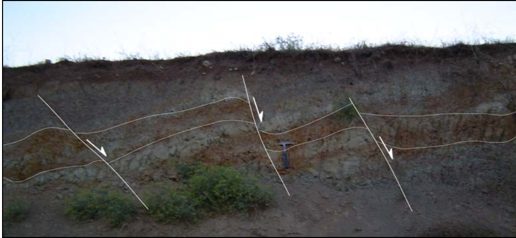
Figure 28. Close-up view of the growth faults exposing on a road cut, within Easkipazar formation (Location: ~750 m SE of Yeniköy, see S 3 on Plate 1 for location).
