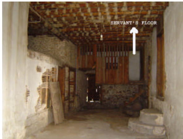
Fig. 143. The Ground Floor and the Servant's Storey in Hacı Güzeller House, Akseki
