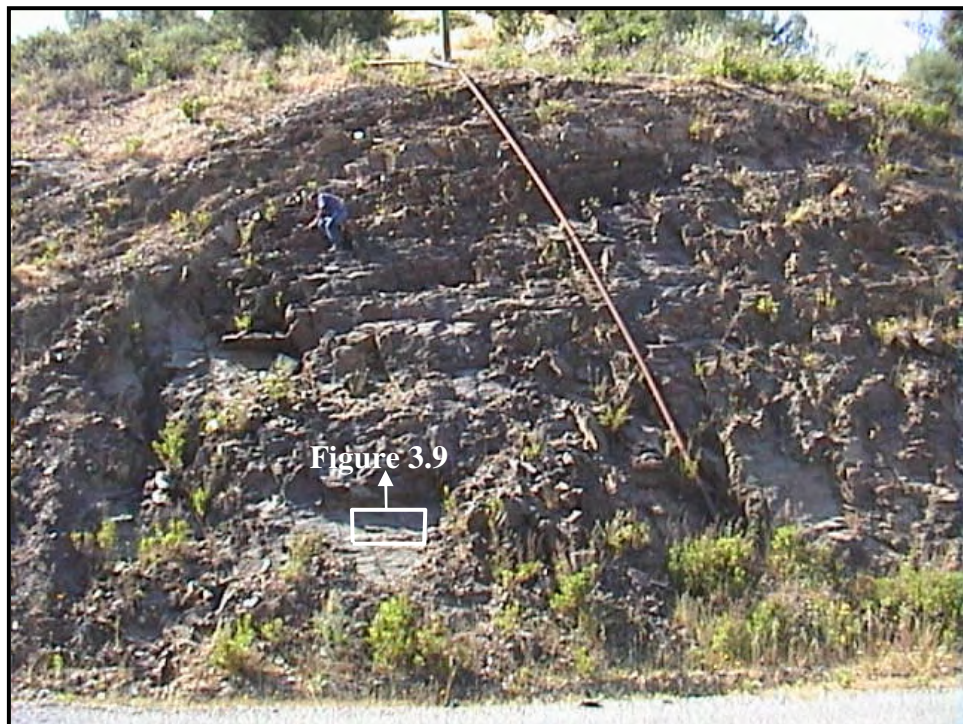
Figure 3.8 General view of schists from the entrance portal of the Dim Tunnel at Km 6+050.
