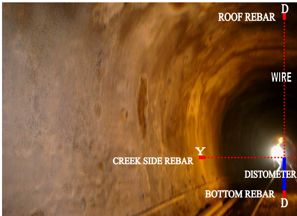
Figure 6.2 General View of a Convergence Station where Horizontal and Vertical Displacements are Measured
