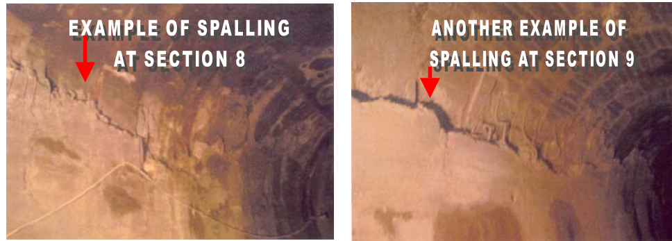
Figure 4.29 Examples of Spalling at the Tunnel before Rehabilitation Work
