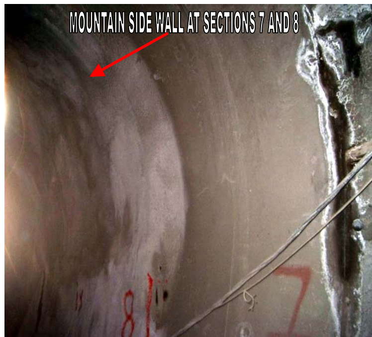
Figure 4.30 The Condition of the Sections 7 and 8 at the Mountain Side after Rehabilitation works
