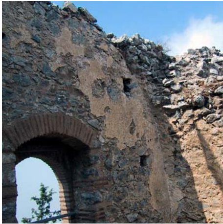
Fig. 158: Plaster Remains On Walls Of The Cells.
