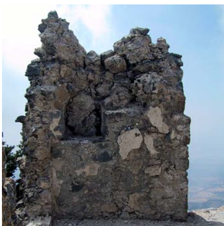
Fig. 162: The Niche In The Room Which May Be An Indication Of A Chapel.
