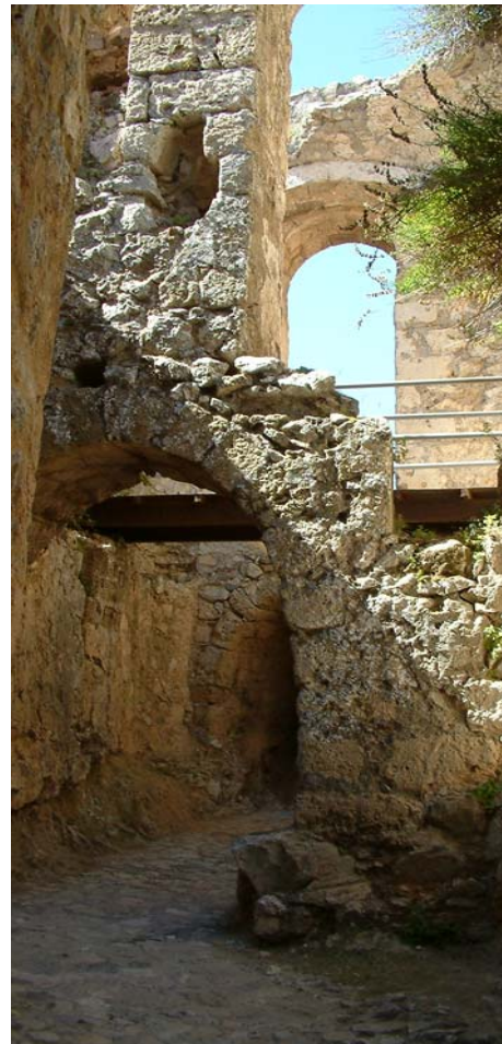
Fig. 118: The Multiple Stories And Different Levels Of The Buildings Of On The First Plateau.
