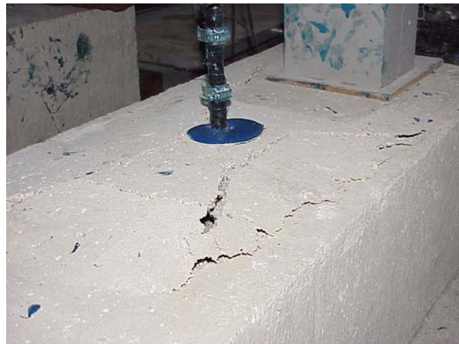
Figure 3.5 Pullout failure of CFRP anchor dowel
