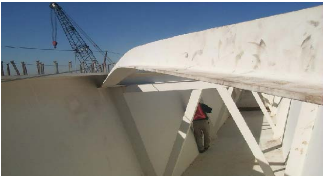
Figure 1.3: Trapezoidal box girder failure during construction
